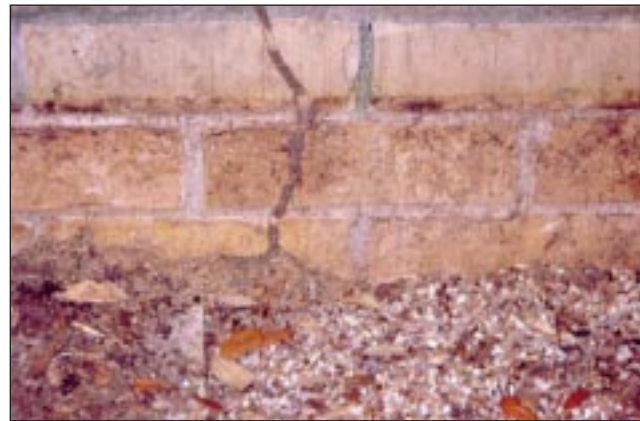
Termite shelter tubes on foundation wall.
