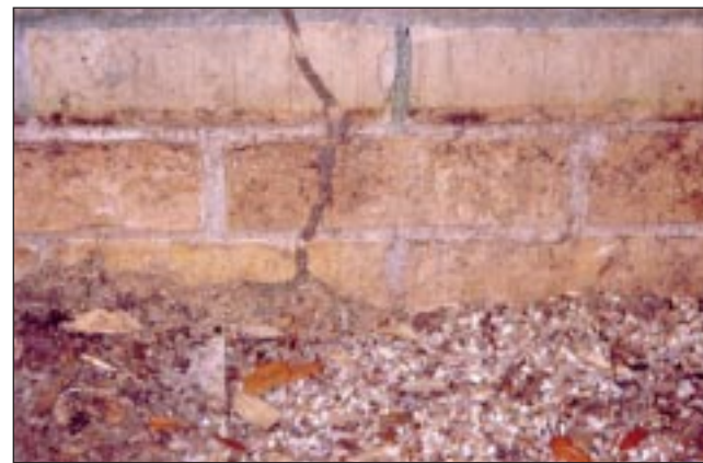
Termite shelter tubes on foundation wall.
